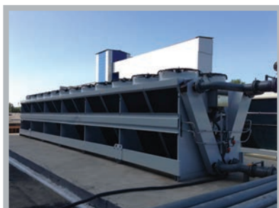
free cooling chillers
