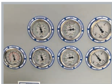
refrigerant and oil gauges
