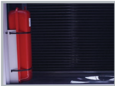
closed expansion tank
