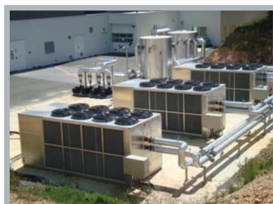
high capacity process chillers
